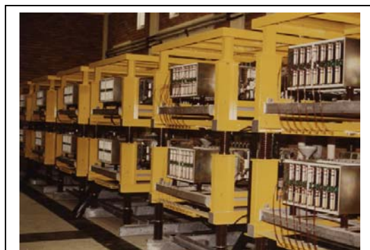
Fig 3 b) for 250 MVar of 400 kV compensator
